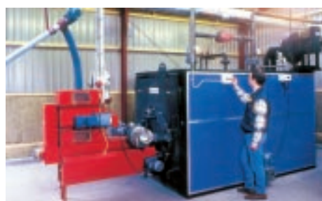
A pelletburner from Danish Linka installed in a boiler with the output of around 500 kW.
