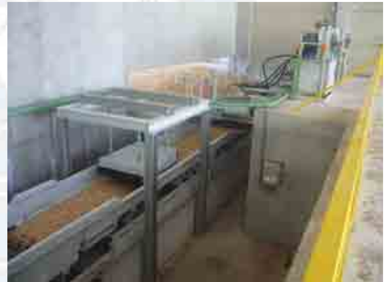
Vibrating conveyor and metal detector
