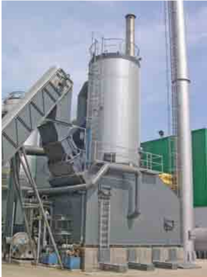
Thermal oil boiler
