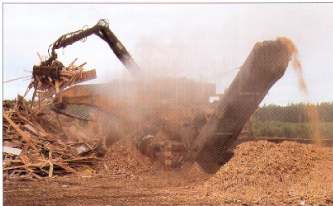
Demolition waste is chipped and incinerated instead of being deposited in a landfill. This is a good way of making use of waste.
