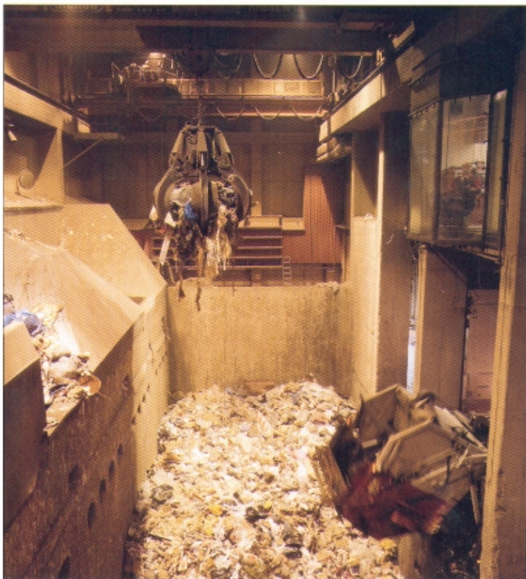
A grab lifts the waste from the bunker and dumps it into the incinerator.
