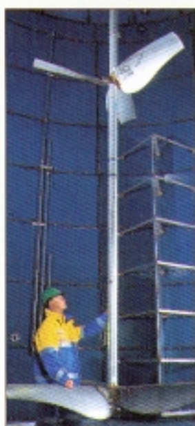
A interior view of the sanitary tank for treatment of the waste before digesting it into fuel for the buses in Linköping. The bio-gas project in Linköping has become a success.
